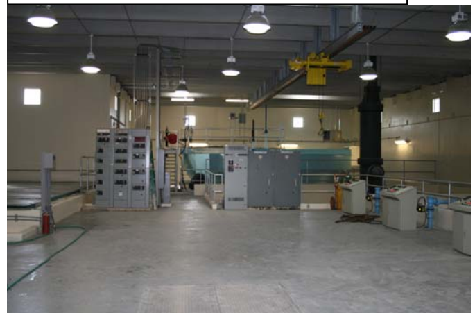
Inside the new East Plant and Claricone Room.
